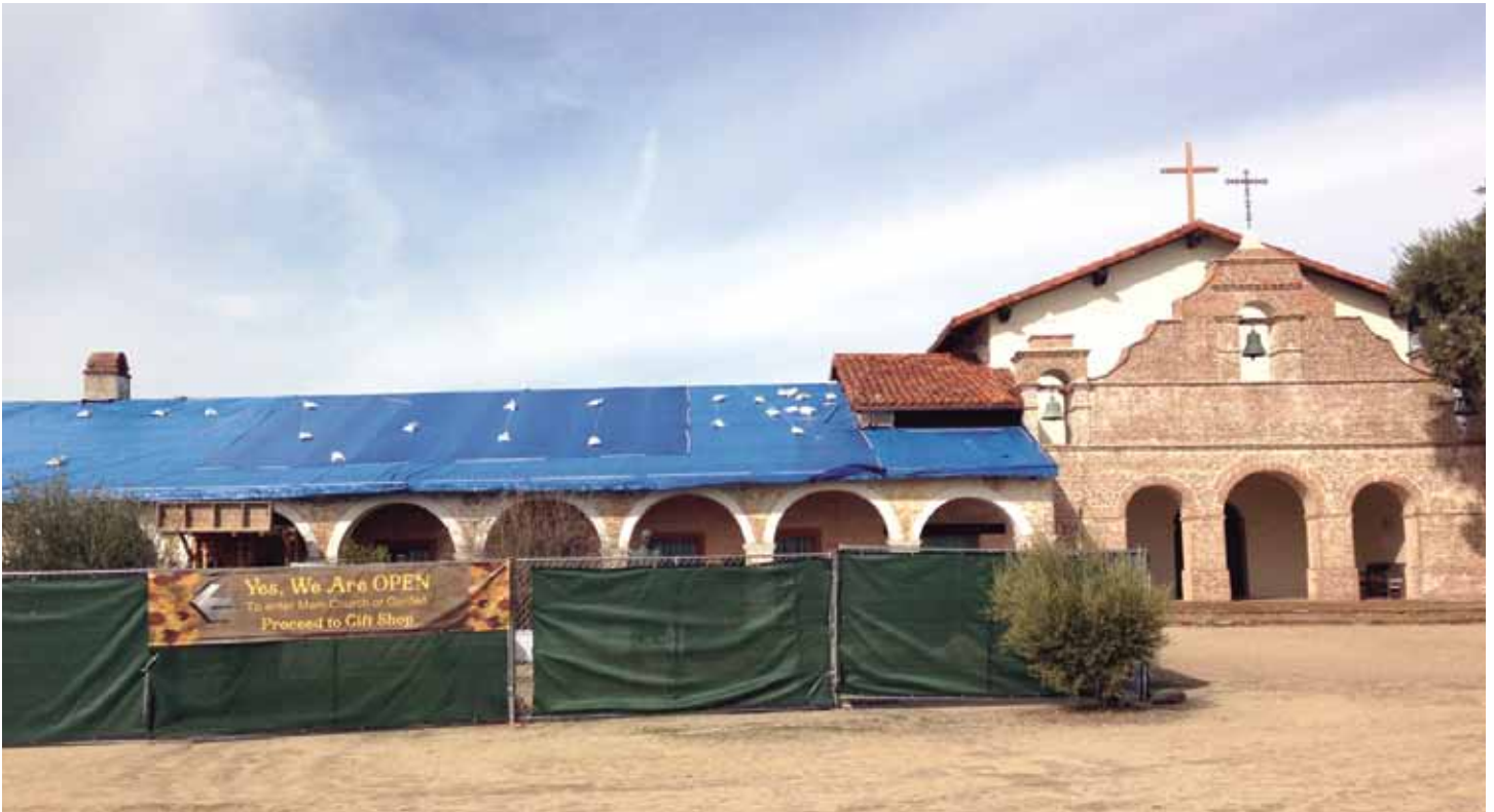
The south convento roof now covered in blue tarps.
