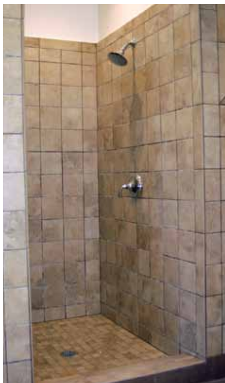
New stall showers in west wing.
