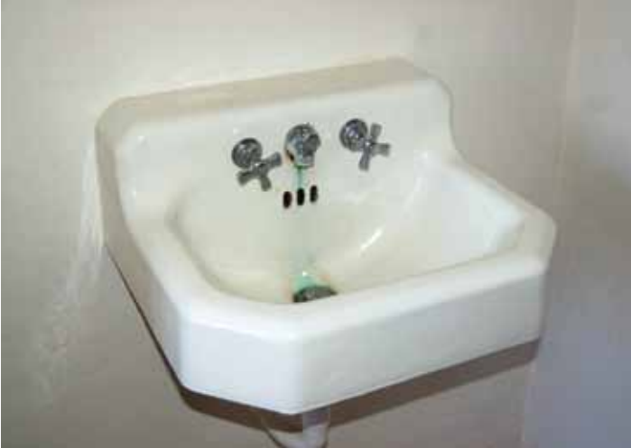
Old sinks in North Convento...awaiting funds to upgrade plumbing.
