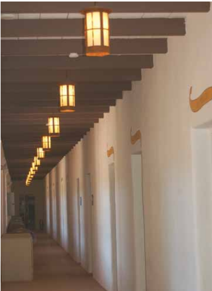
North Convento retreat center with electrical upgrade and new motion-sensor lights. Emergency lighting is also in place now in the retreat center corridors.
