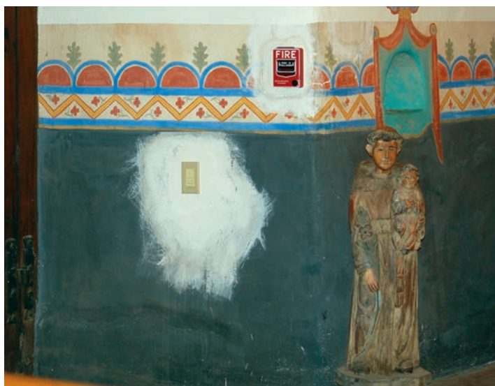
"Before" picture of an area of the church in need of paint restoration.
