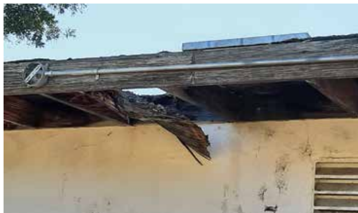
The building was definitely showing signs of major distress and unsafe conditions.
