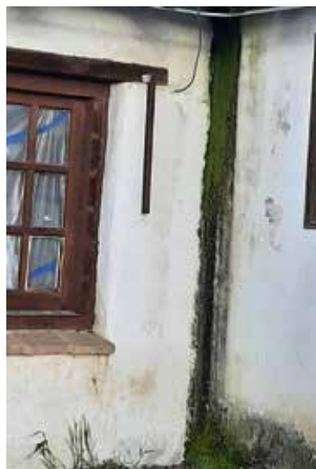
Conditions of the building became increasingly unhealthy and unsafe after a water disaster in 2014.
