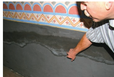
Picture of efflorescence present on the East interior wall of the church. Also referred to as a "Tide Line" indicating water penetration into the wall, and subsequent escape.
